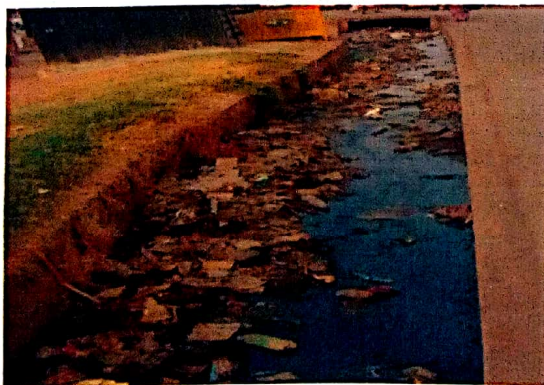
Plate 1.4: Blocked Drainage in Zone M.
