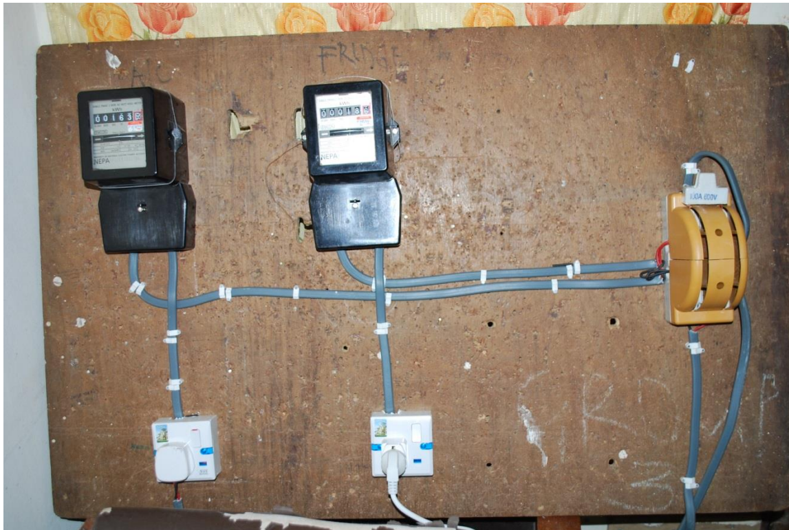
FIGURE 7.12: INSTALLATION OF METERS FOR THE EXPERIMENTAL
