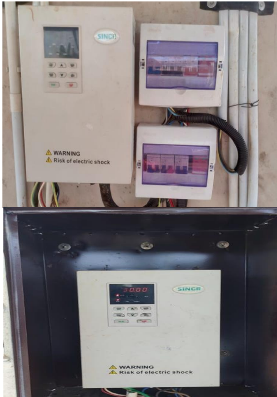
Figure 11: Solar pump inverter during operation.
