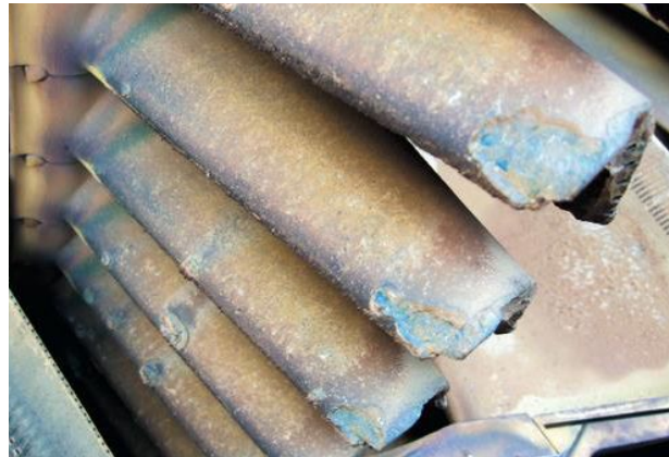
Plate 1: Degraded turbine blade tips (Bacos, 2011)
