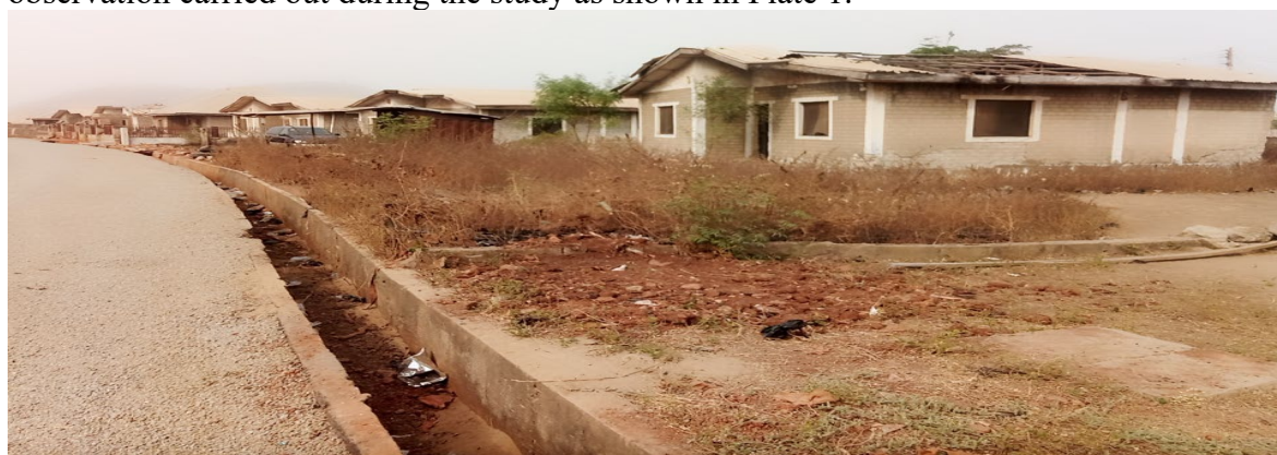
Plate 1: Wall and Roof Conditions of Harmony estates Ilorin Source: Authors' field survey, (2021)
